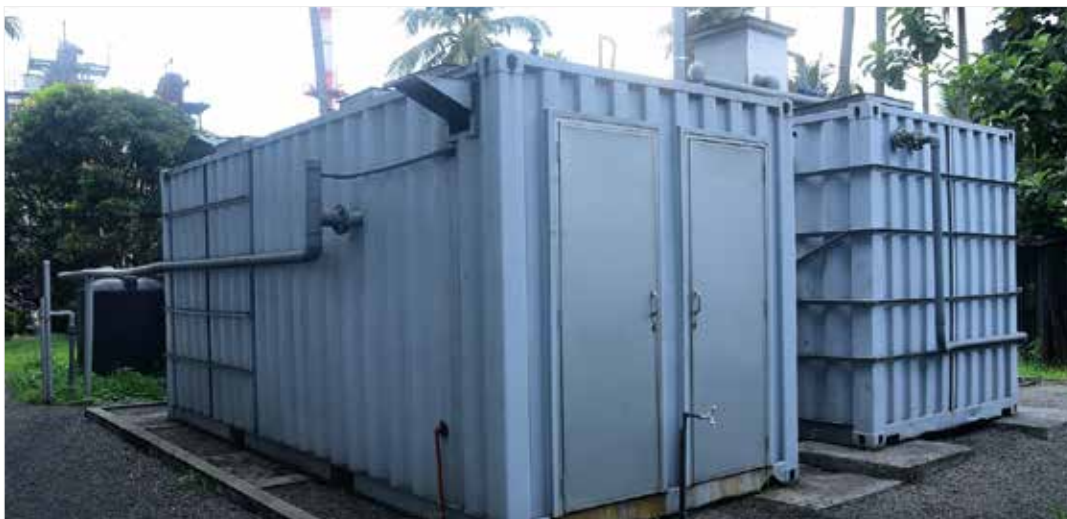
Containerized wastewater treatment system
