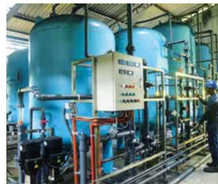
Deionised water plant
